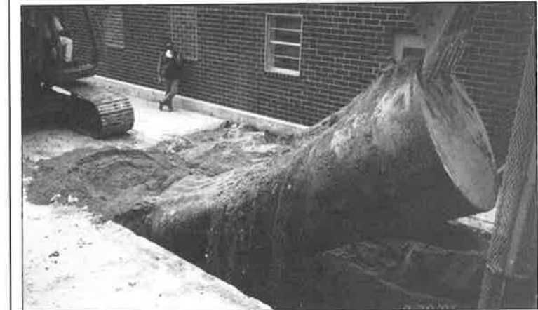
Digging up the past – after 25 years, workers removed the old diesel storage tank.
